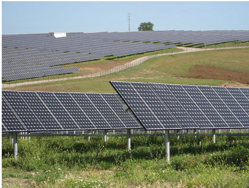
Figure 3.6: The 11 megawatt Serpa photovoltaic installation in Portugal.
