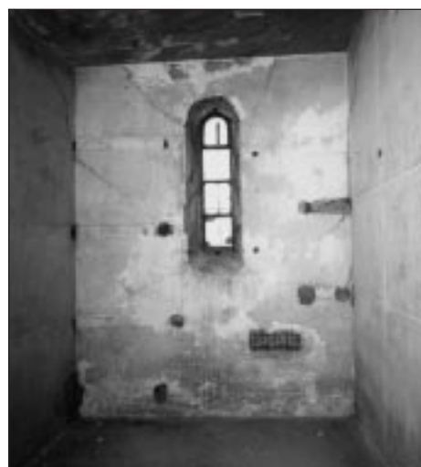
One of eight prison cells where conscientious objectors were imprisoned during the First World War. The graffiti written by these prisoners still survives on many of the fragile lime-washed walls.
